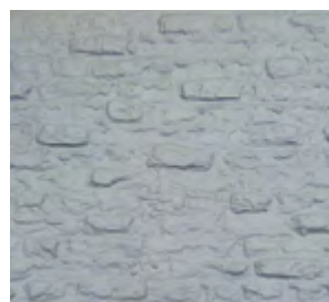
Rough Worn Brickwork
